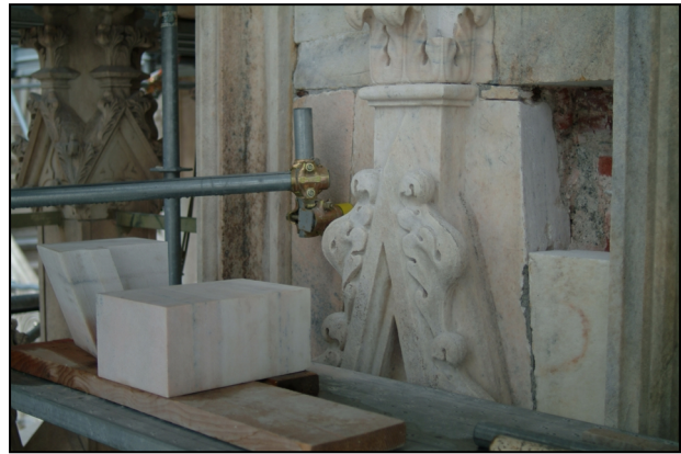
Figure 14. Replacement of a damaged marble block on a counterfort of the Façade during the restoration.
